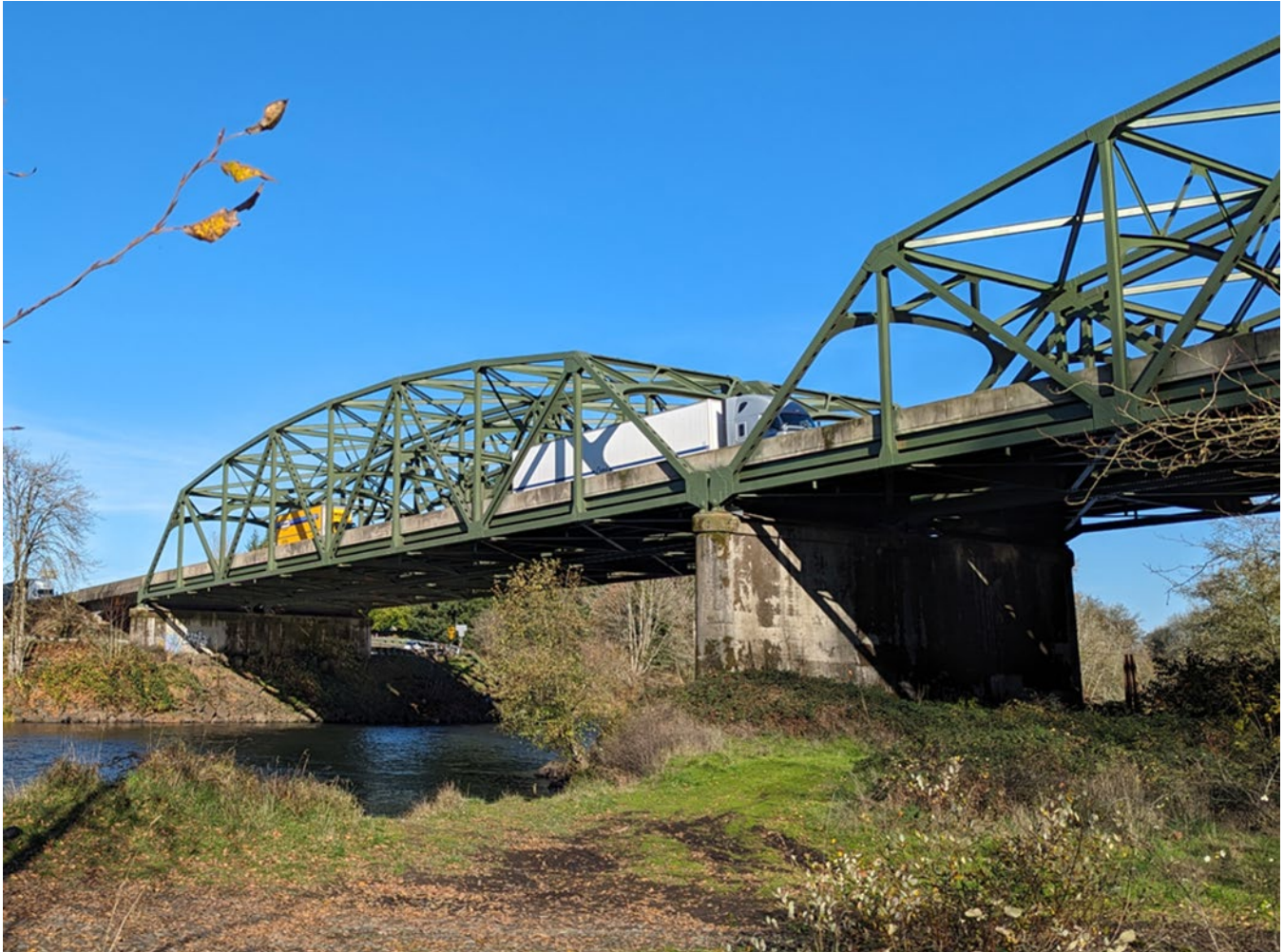
Figure 5-14. Existing bridge over the Cowlitz River; photo taken from south (river-left) bank looking north.
