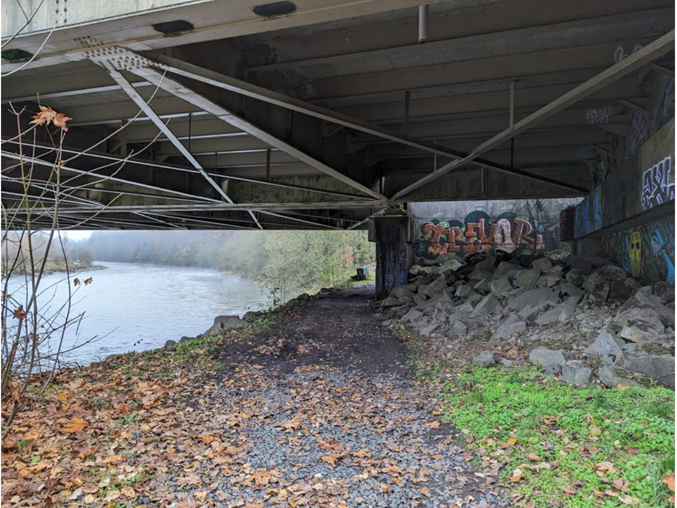
Figure 5-5. Trail on south (left) bank of Toutle River under the southbound bridge.
