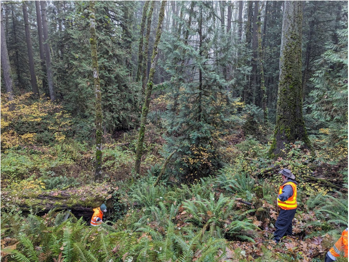
Figure 5-8. Channel downstream of the MP 53.9 culvert (culvert outlet not located during site assessment).
