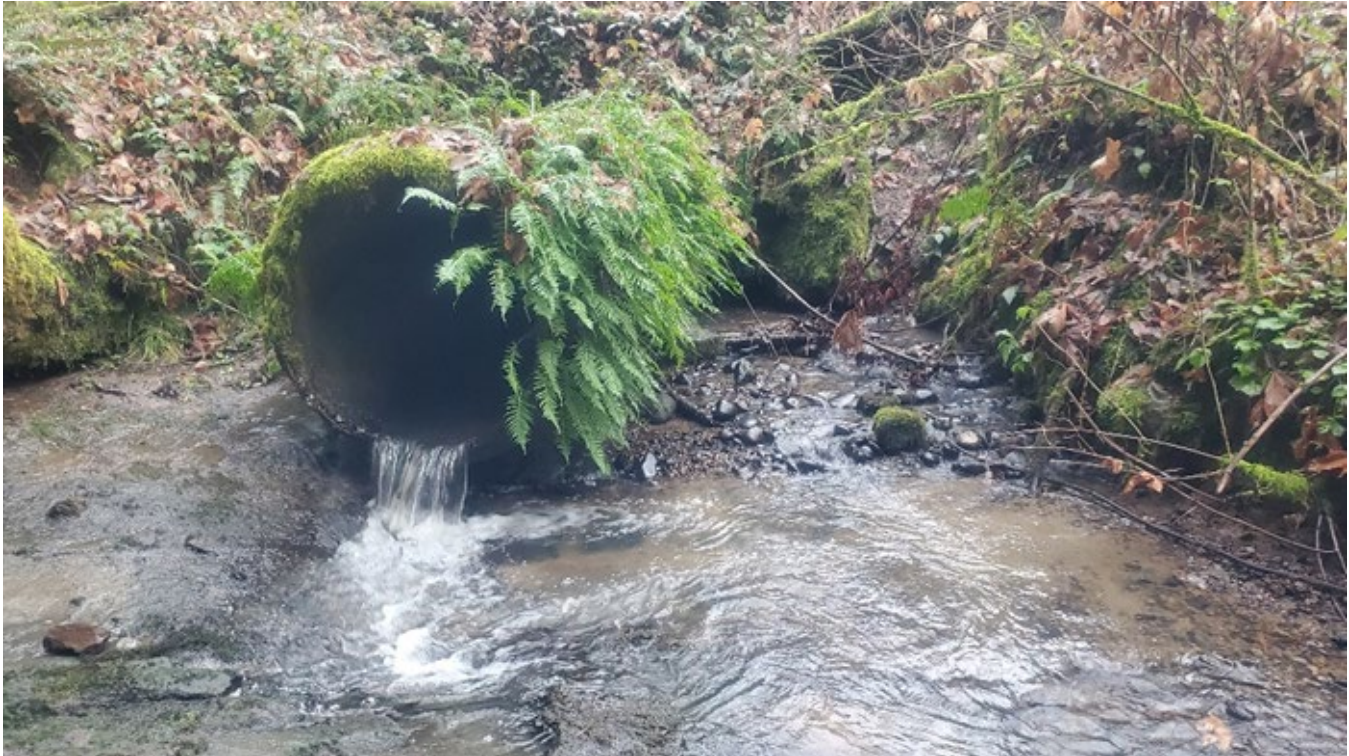
Figure 5-7. MP 53.07 UNT Cowlitz River culvert outlet from December 2023 WSDOT fish passage assessment.
